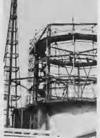
SAFETY OF total plant operation is depicted by the re-construction of an inert gas tank near Alky-2. SEGURIDAD di operacion total ta ilustra door di re-construccion di un tanki di gas inactivo.
